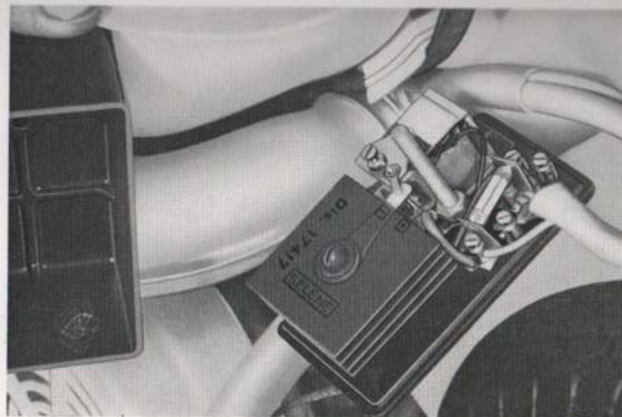
Relay unit and large half-wave rectifier. Note 5 amp. fuse
